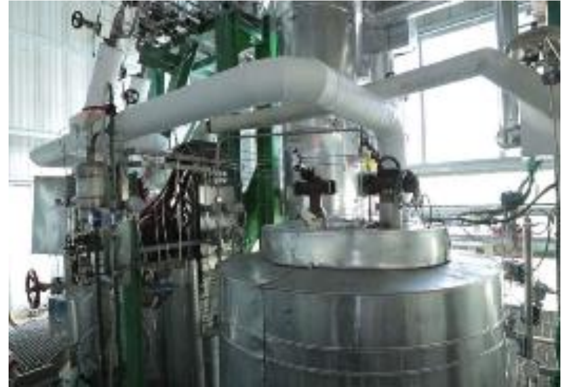
CSG steam generator performance experimental validation Temperature & pressure thermohydraulic testing (2019)
